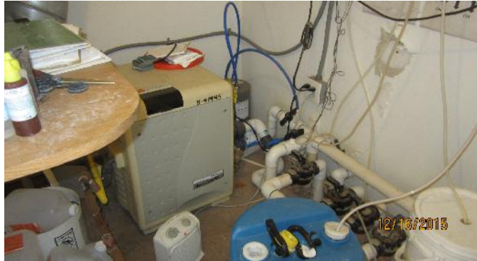
The pool heater was replaced in 2013. The useful life is 6 years per meeting.
